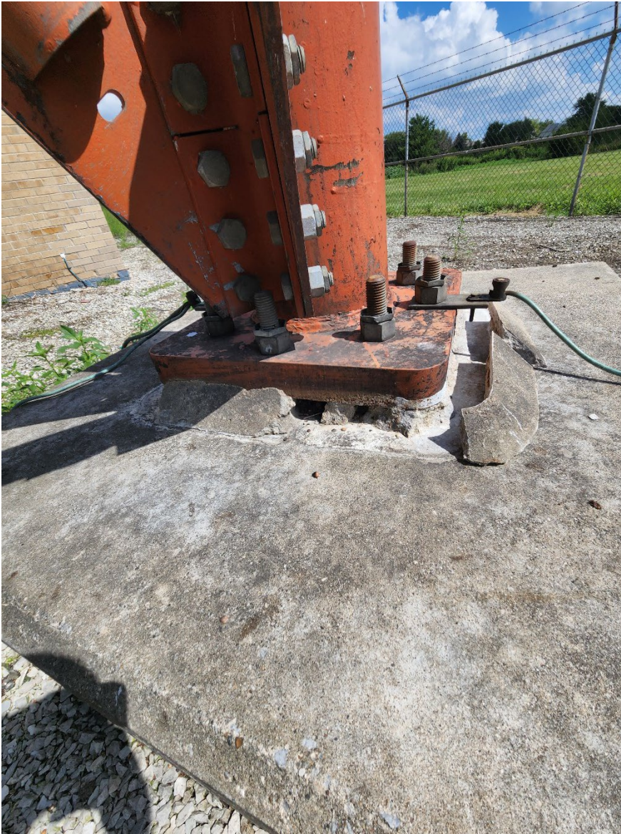
Issue 4 Grout needs repair
