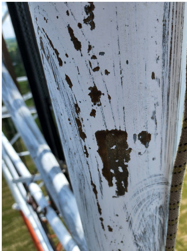
issue 2 – paint condition poor
