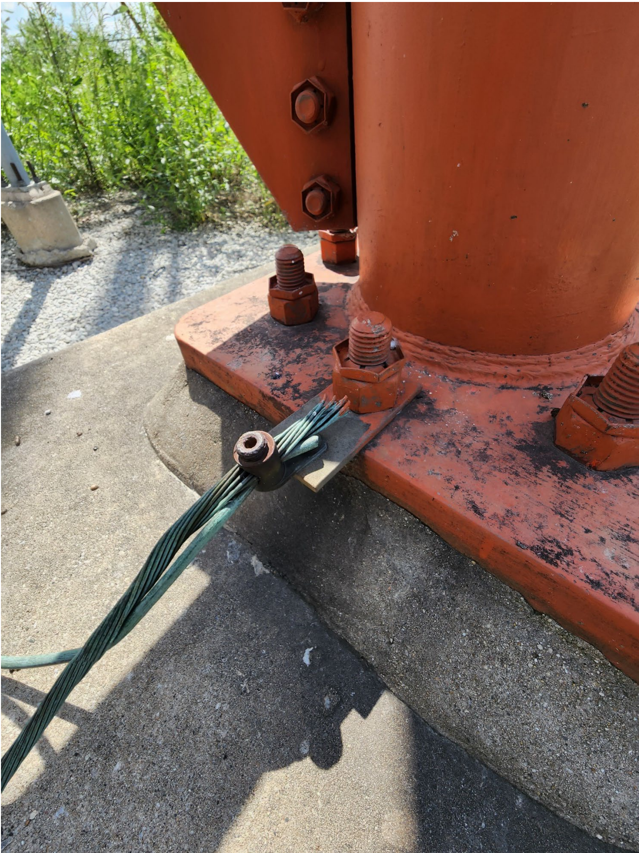
Issue 3 – base grounds needs to be cadweled
