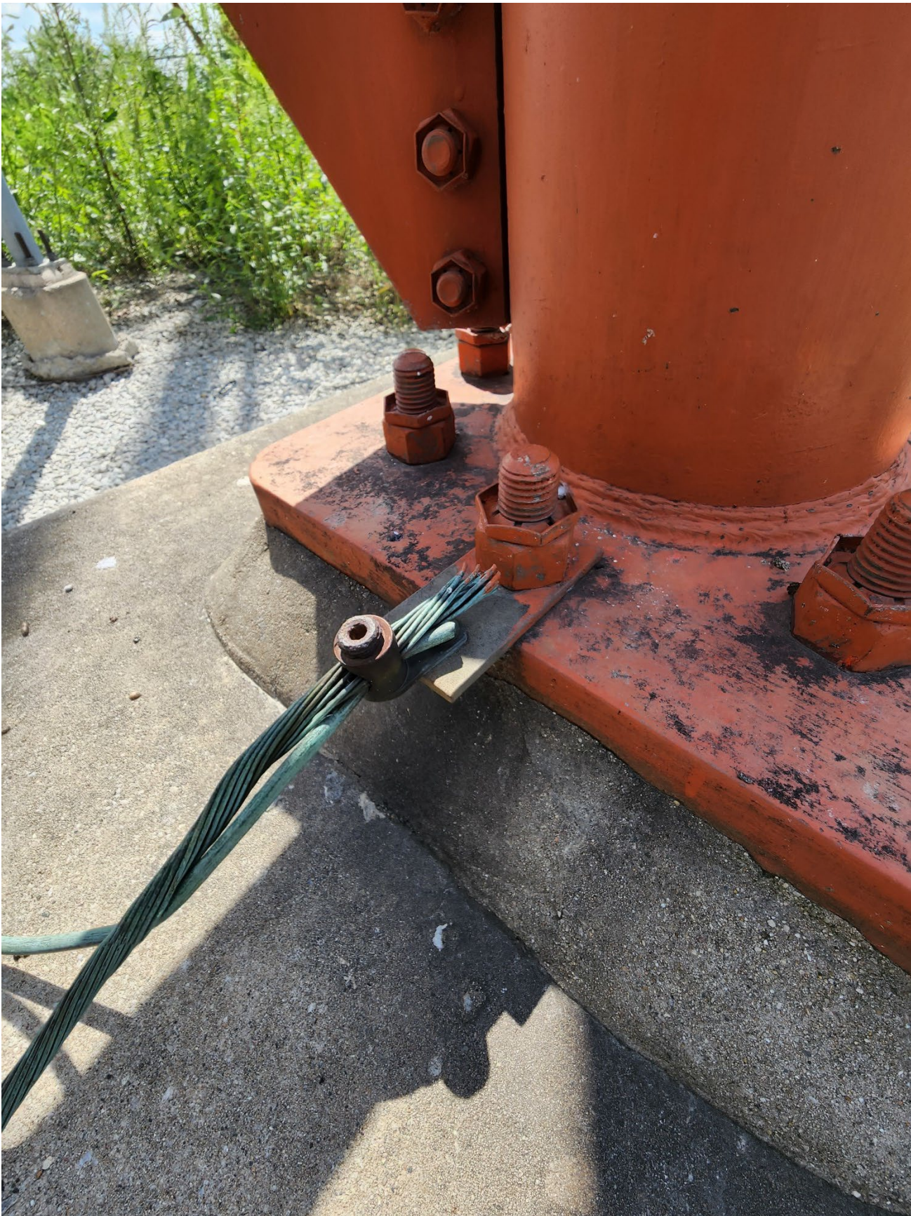
Issue 3 – base grounds needs to be cadweled
