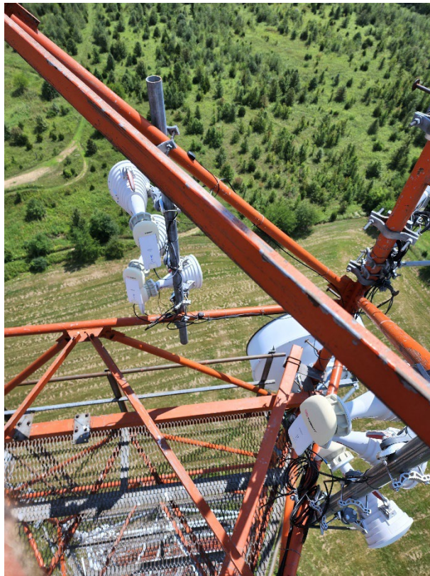
Issue 6 wi fi clamps should be replaced
