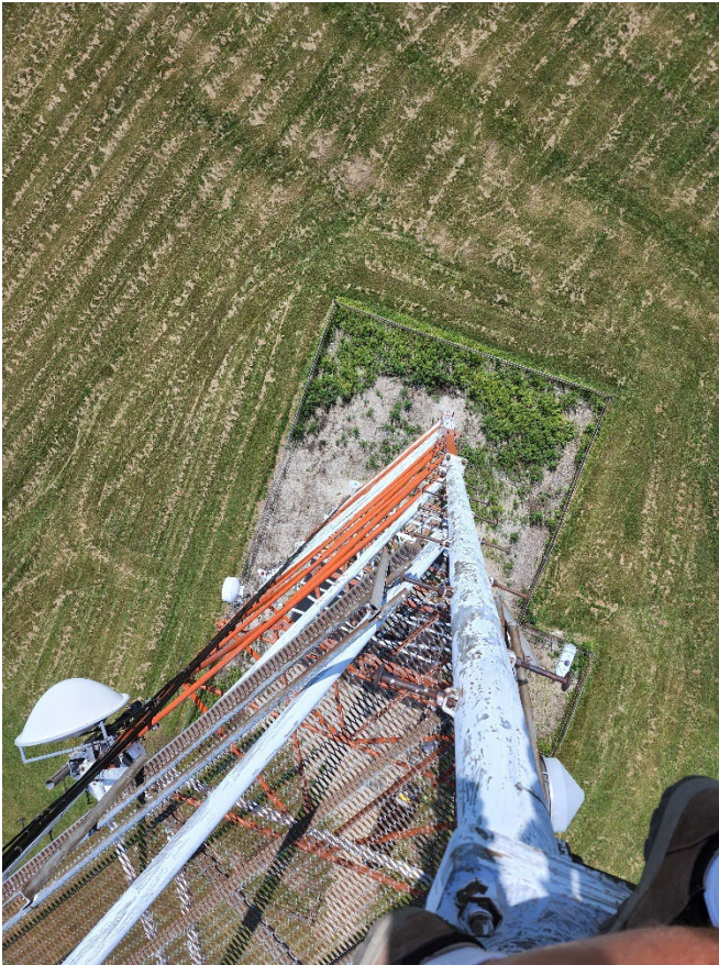
Paint condition poor
