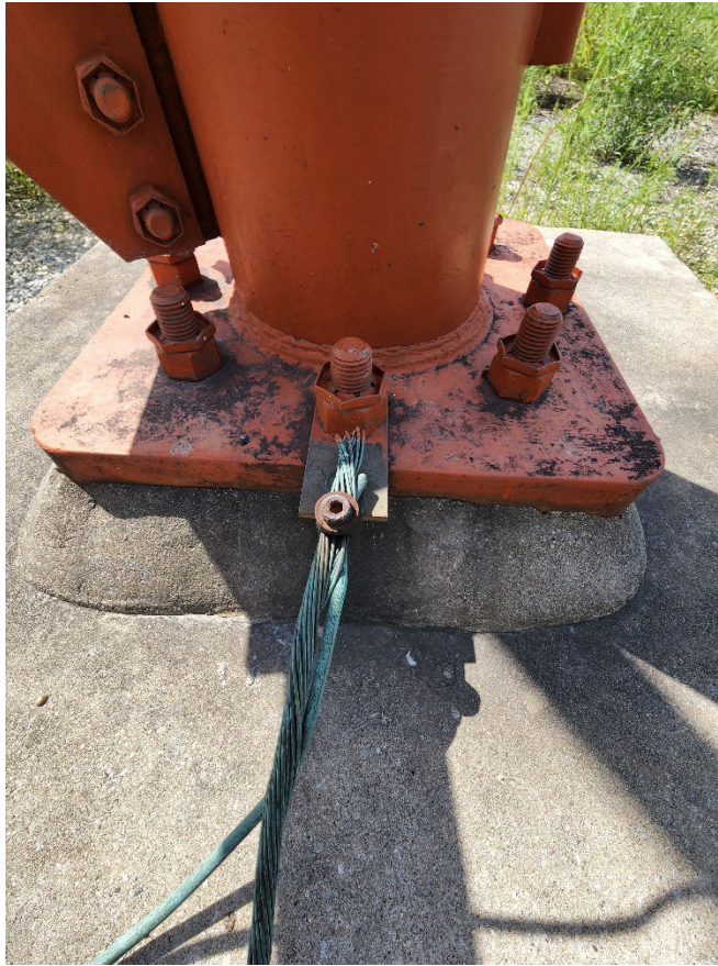
Issue 5 Anchor bolt inspection, water could be getting trapped
