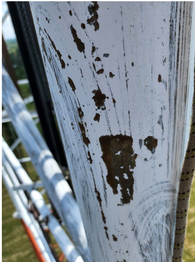
issue 2 – paint condition poor
