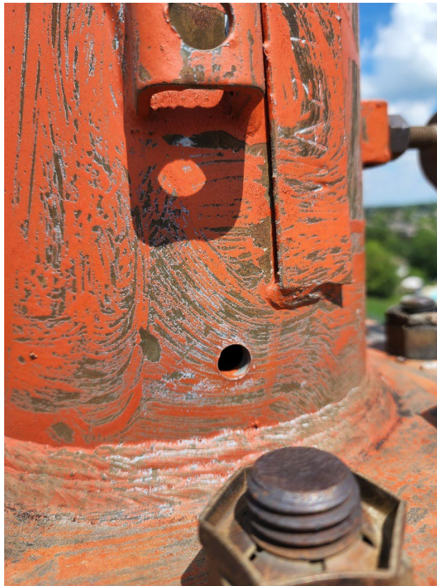
Paint condition is poor, galvanized rust bleed & hardware rust is plentiful
