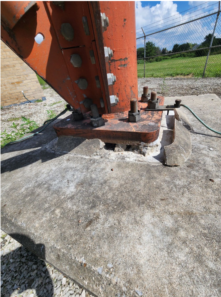
Issue 4 Grout needs repair
