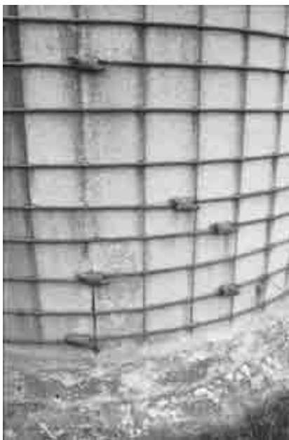
Above: A detail view of the steel hoops and turnbuckles on a concrete stave silo. Right: An advertisement for concrete stave silos from the Prairie Farmer's Reliable Directory (1918), 359.
